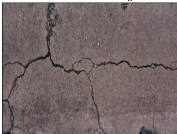
Figure 2: The crack on concrete due to the low tensile strength Source: Raza et al., (2020).
