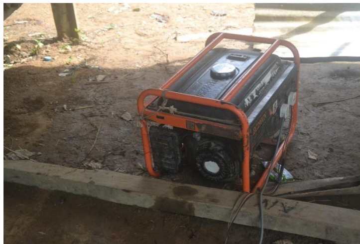
Figure 4: The Diesel Generator to Get the Power Sources at the Village
