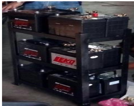
Figure 4: Solar power controller
